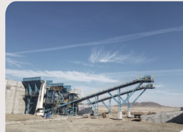
650 t/h Mining Project, Karaganda, Kazakhstan, SCADA automated
