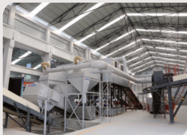
300 t/h Construction Waste Recycling Project, Guangdong, China
